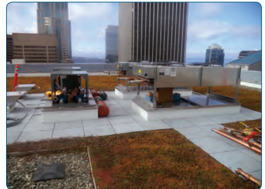
Above: The new cooling system takes air from the outside and filters it into the server/network room at much lower cost than the previous air conditioning units.
